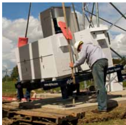
1,320W Hybrid Power System with solar, generator and battery power
