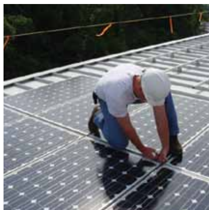
Used 5,880 solar panels
