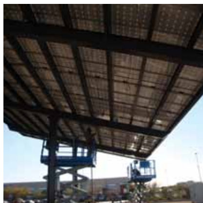
Will generate more than 32,000kWh per year
