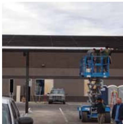
Used 120 solar panels
