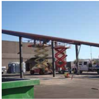
Alpha designed the elevated solar racking structure
